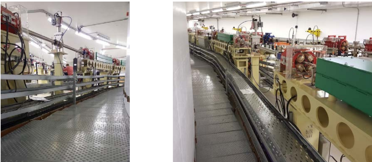
Figure 2-152 : Booster Vault showing the cable containment inboard of the booster ring.
