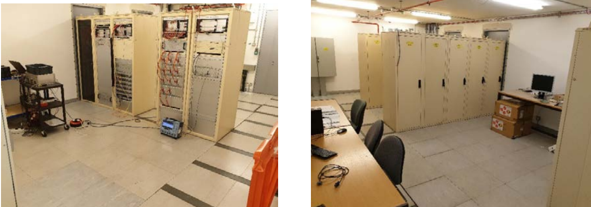
Figure 2-154 : Booster CIAs 1 & 2 showing spare rack positions.
